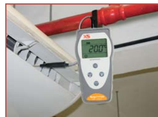
Temperature measurement in air conditioning system
